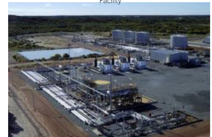
Arrowsmith Stabilisation Plant – Future CO2 Aggregation Facility
